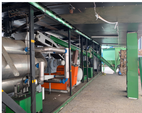
Regreen Technologies Inc. Total Waste System located at Hesperia in California.
